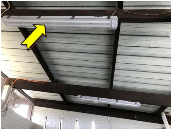
Photo 3. Interior, throughout, double tube fluorescent light fitting – suspected PCB-containing capacitors.
