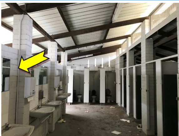
Photo 5. Interior, throughout, walls – suspected lead-containing white upper paint systems.
