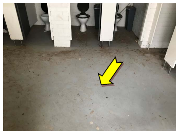
Photo 6. Interior, throughout, floors – suspected lead-containing grey upper paint systems.
