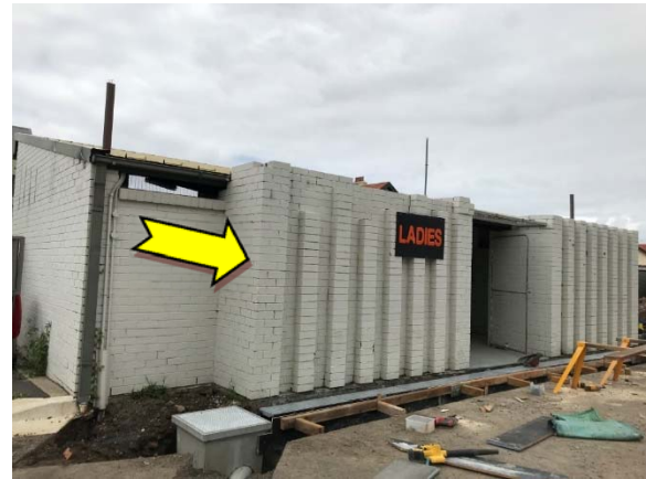
Photo 4. Exterior, throughout, walls – suspected lead-containing white upper paint systems.
