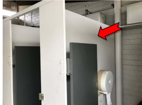
Photo 2. Interior, cubicle, side partitions – asbestos-containing compressed cement sheeting.
