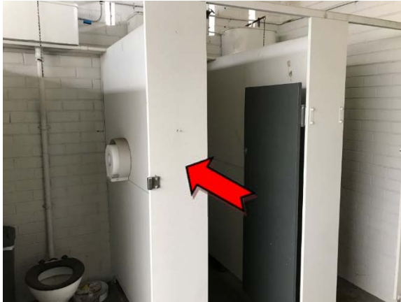
Photo 1. Interior, cubicle, front partitions – asbestos-containing compressed cement sheeting.
